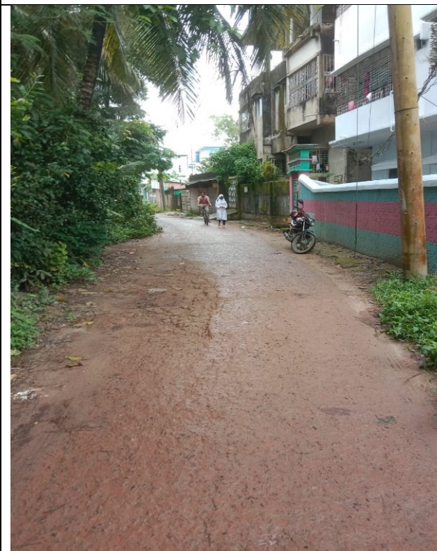
Photo SP.RD8.002: Existing Damaged RCC Road
