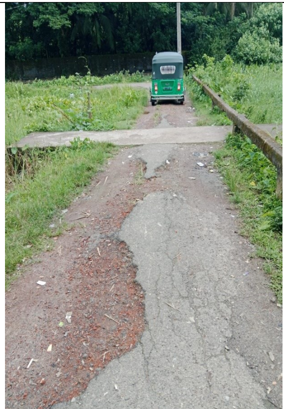
Photo SP.RD7.001: Existing Damaged BC & RCC Road
