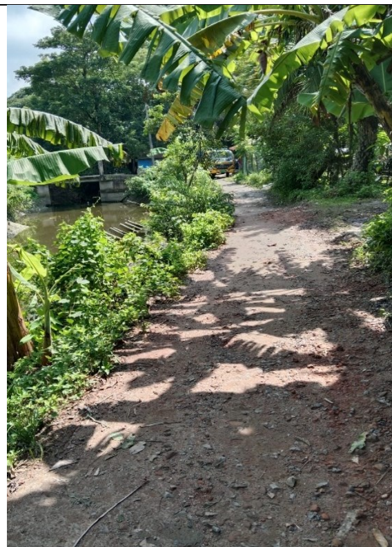
Photo SP.RD9.002: Existing Damaged BC Road
