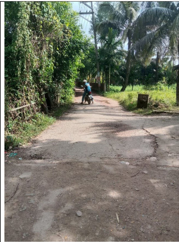
Photo SP.RD3.001: Existing Damaged BC Road
